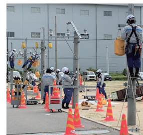
Power distribution training
