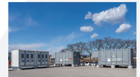
Storage system in the Kameokacho district of the city of Ota
