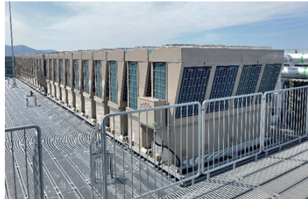
ES Business Rooftop Equipment, Main Building, Fukuoka University Hospital Energy
